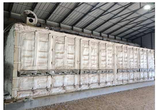
Image 1: Closed Carbonation Chambers.
